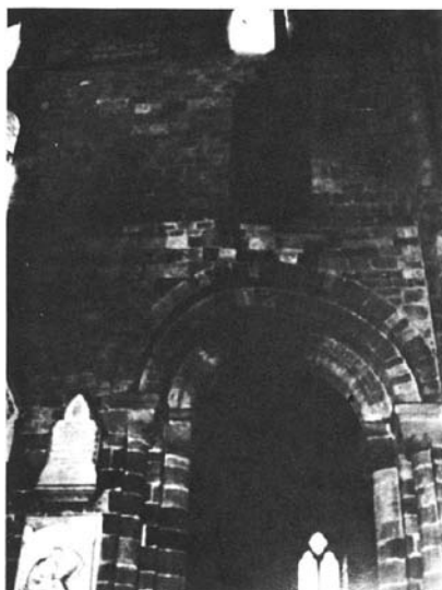
Fig. 67 An arch deformed by subsidence in Carlisle Cathedral. No movement seems to have occurred after about 1300–50. Compaction of the site through drying out of the soil in the previous centuries has been suspected as the cause of the damage seen (see pp. 197–8).
